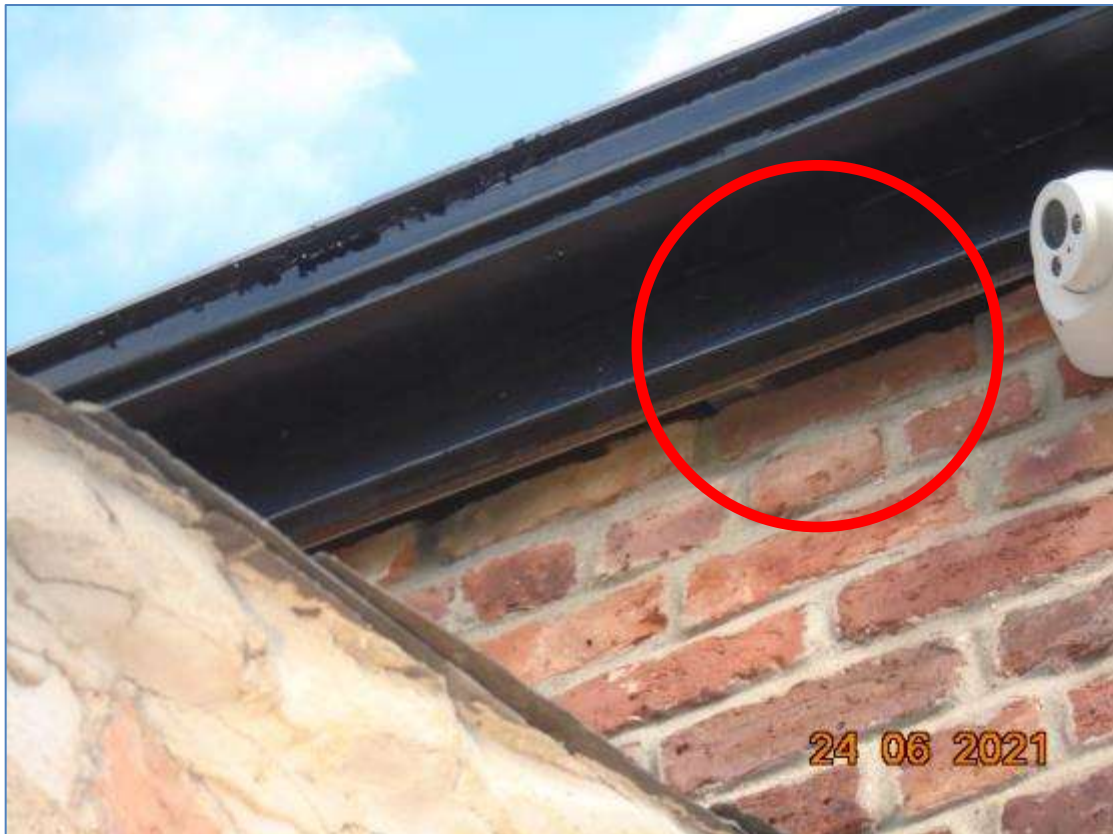
Photograph 4 – Fascia gaps on the rear (south) elevation.
