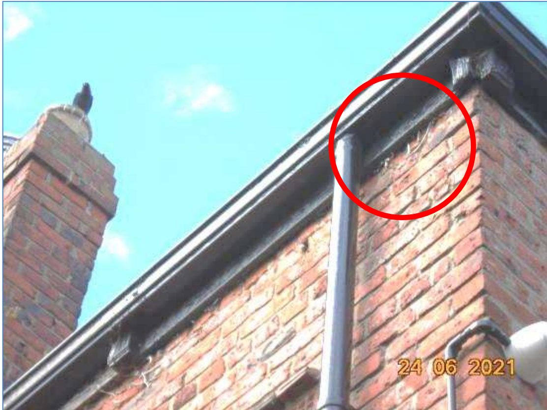
Photograph 3 – Fascia gaps on the side (east) elevation.
