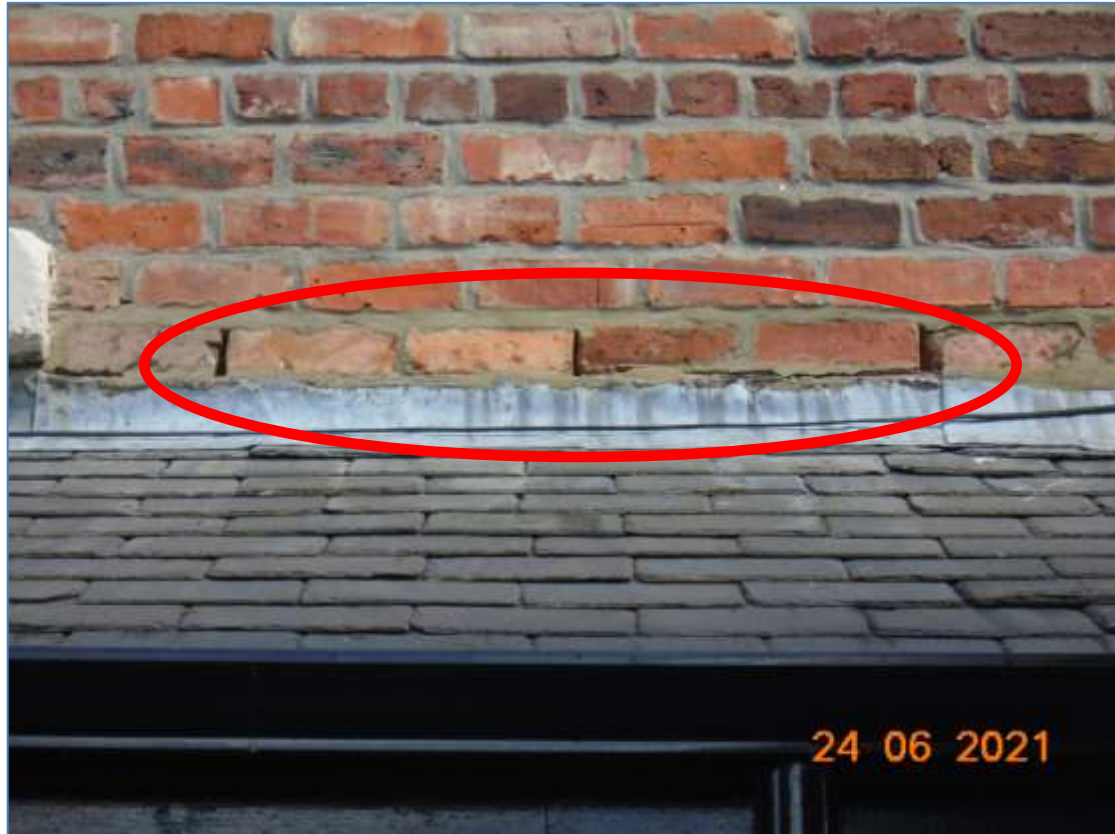
Photograph 5 – Brickwork mortar gaps on the rear elevation.
